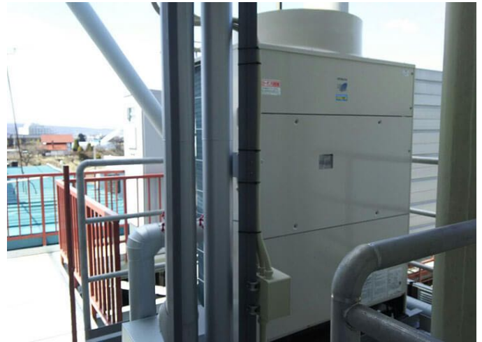
Chillers in Karuizawa plant
