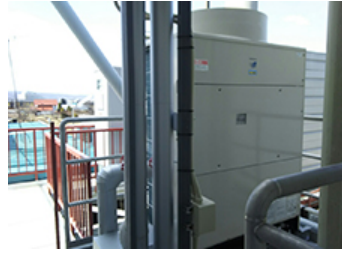
Chillers in Karuizawa plant
