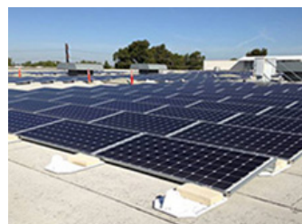
Santa Ana Plant
