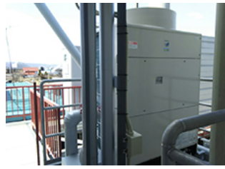
Chillers in Karuizawa plant
