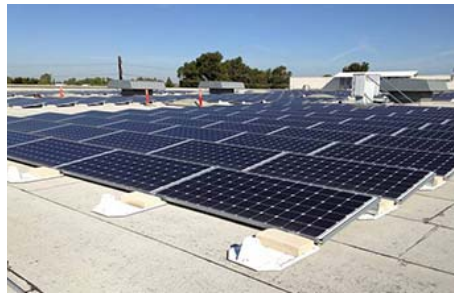
Santa Ana Plant
